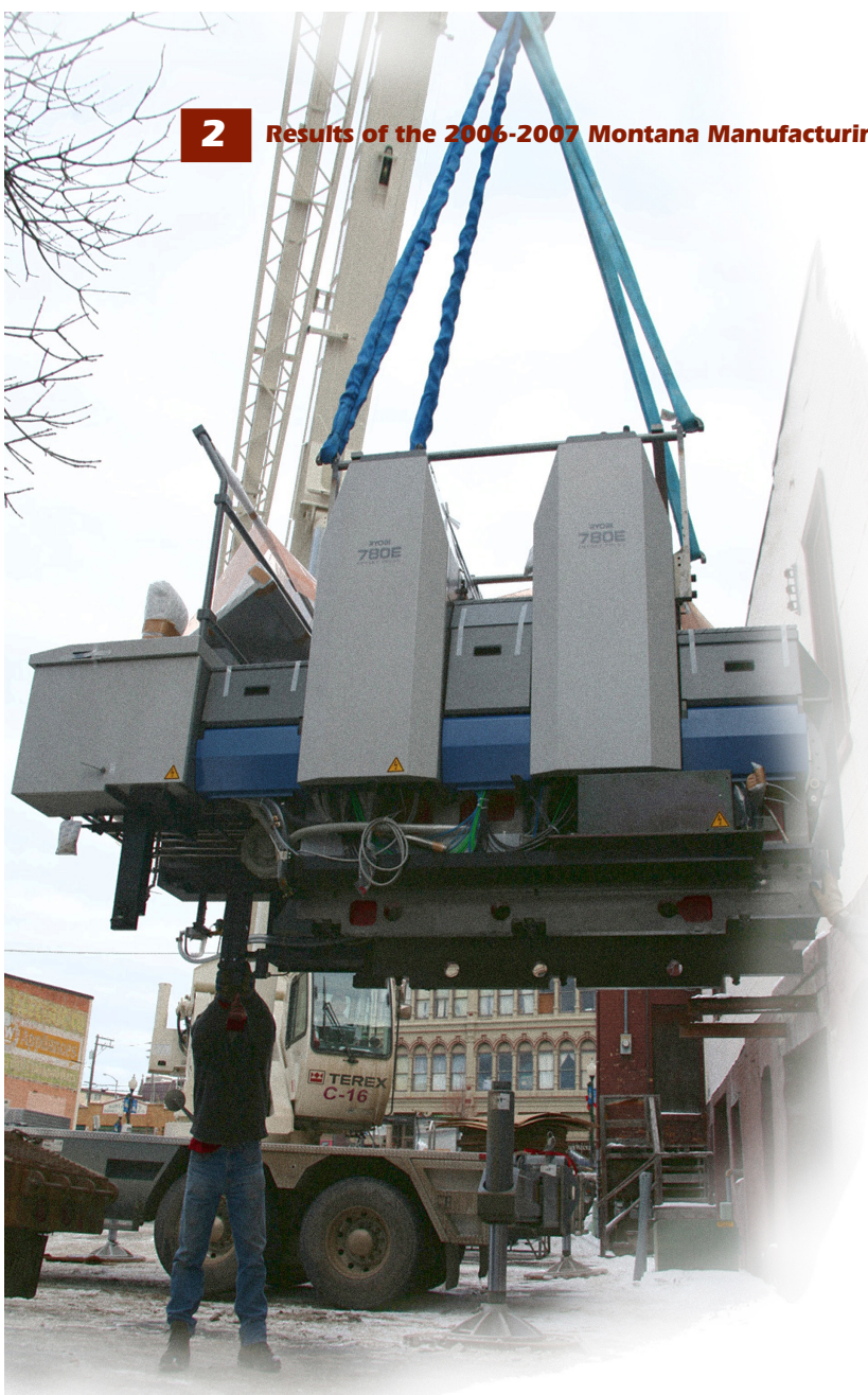
Printing press being readied for installation at Allegra Print in Helena. Photo by Archie Broadbent. On the cover: skilled welders are one example of the needs in the manufacturing workforce.
