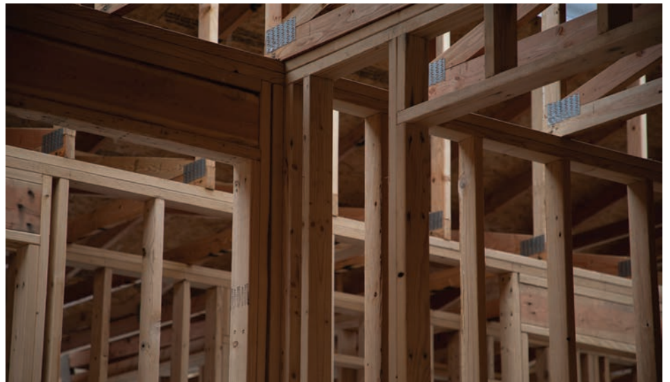
Finished framing on the inside of a house being built by the Sustainable Construction program at Missoula College. Photo courtesy of University of Montana.
